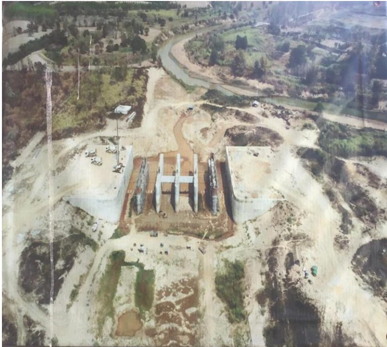
Figure 2: The Picture of the KCR Construction Site on Baan Sao Wa wetland Forest (Source: Researcher, 2021)
