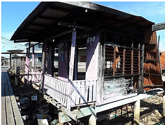
Figure 2 House burnt down condition By: Punya Tepsing, 27 July 2016
