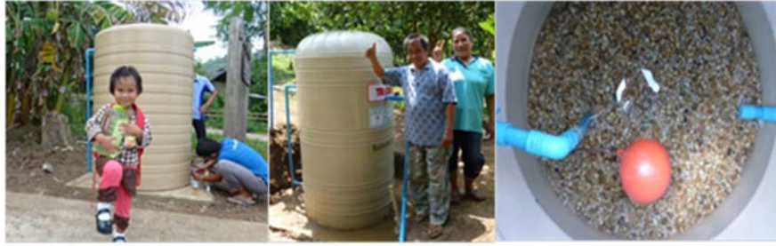
Figure 8 Pilot site of Slow Sand Filter for drinking water, at village 4
